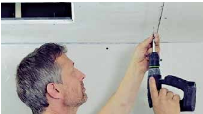
and screw the drywall sheet into the ceiling. Seal the cable hole in the back box.
