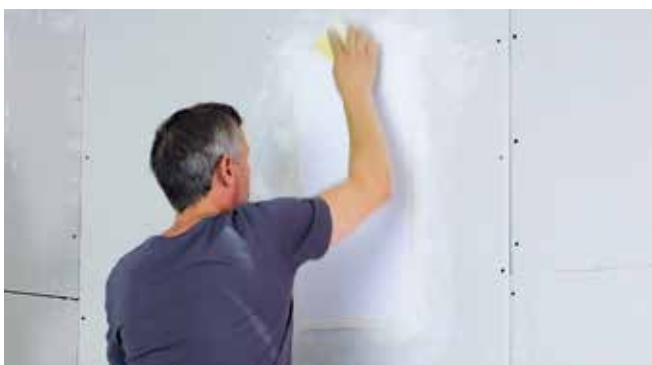
Sand off excess filler. ATTENTION! The primer on the membrane must not be sanded through!
