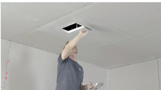
Fill the edges. Be sure to remove the filler from the inside.
